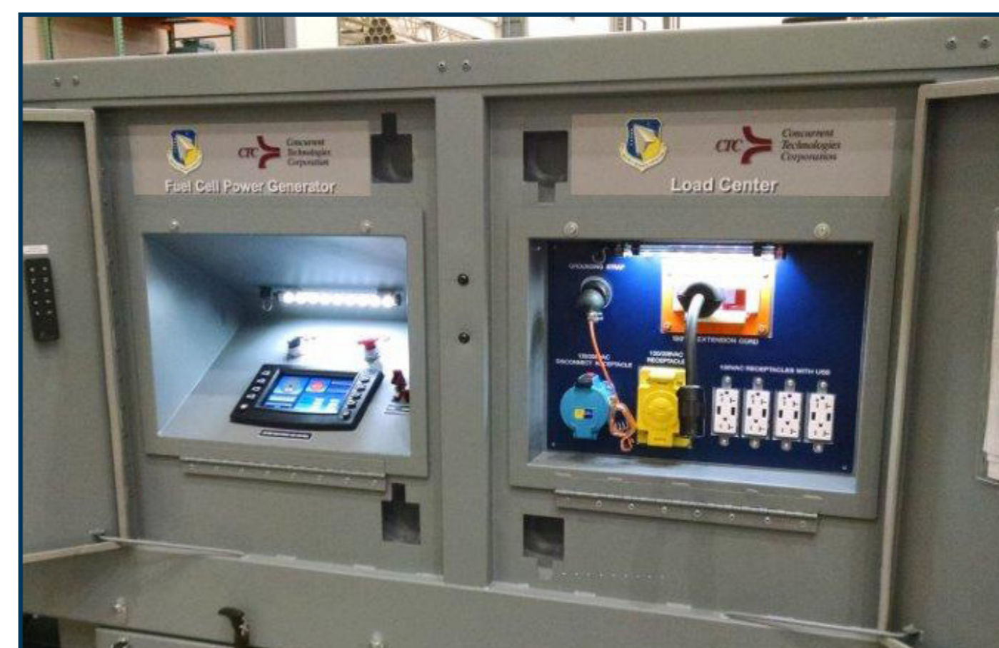
Control Panel / Load Center
